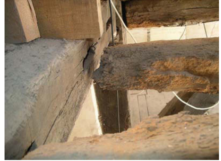
Fig. 1 Detached floor joists
