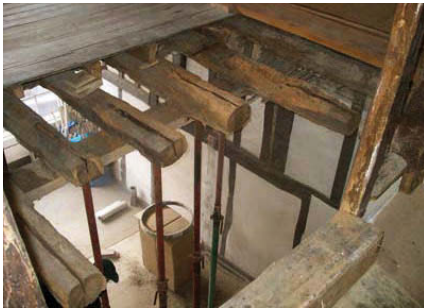
Fig. 2 Propped floor joists with decay removed
